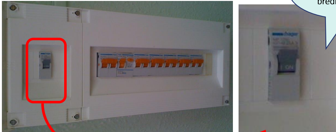
Example 2. Circuit Breaker Box and Close-Up of the Main Breaker
