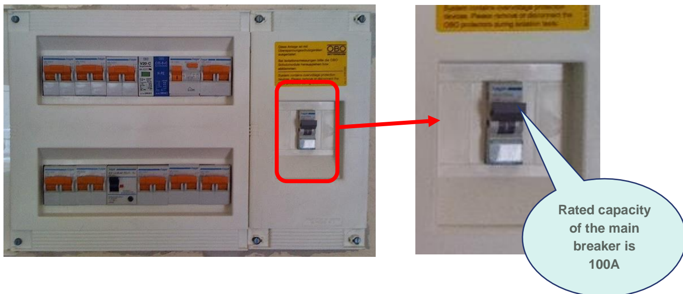
Example 1. Circuit Breaker Box and Close-Up of the Main Breaker
