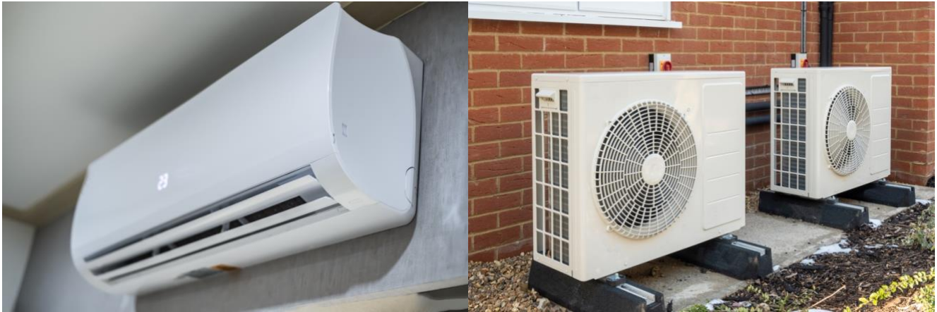
Left: “Mini-split” or “multi-split mounted air handler. Right: Outdoor heat condenser.
