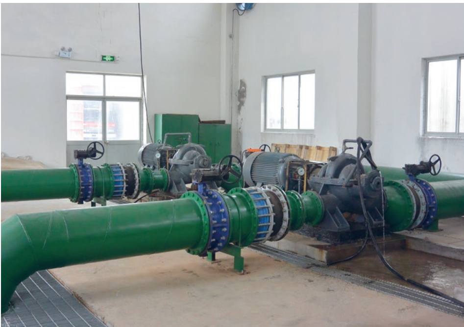
Figure 5: Pumping System in a Chemical Processing Plant (Source: Impact Energy AG, 2014)
